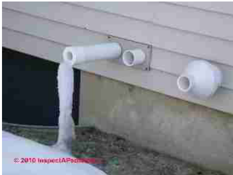
Exhaust pipe blockage of ice and snow can cause carbon monoxide to build inside the home. Image Source: http://inspectapedia.com
